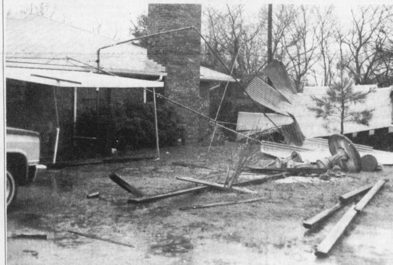
DESTROYED -This tractor shed belonging to James Norwood of Cunningham was blown away and
