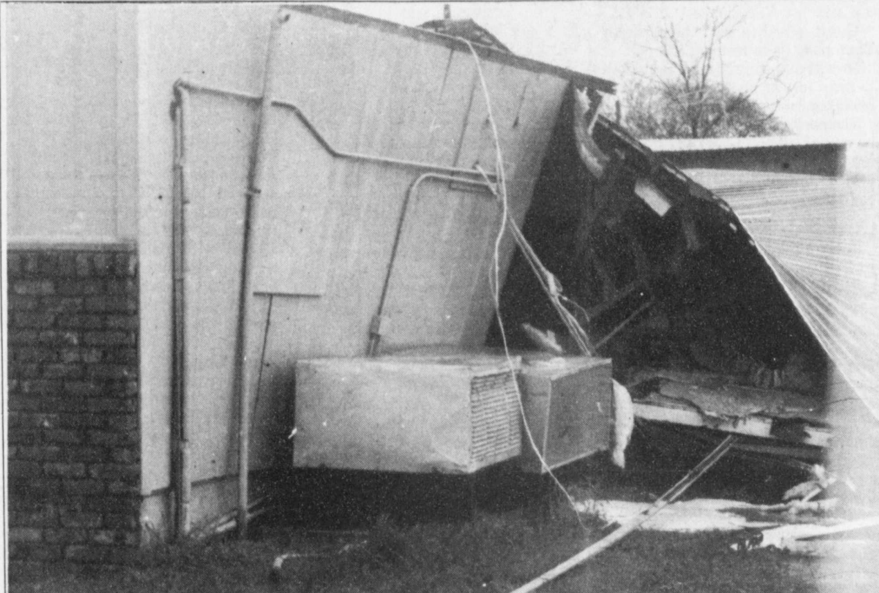
DESTROYED -Quickie Superette in Deport was destroyed by the tornado that struck in the early
