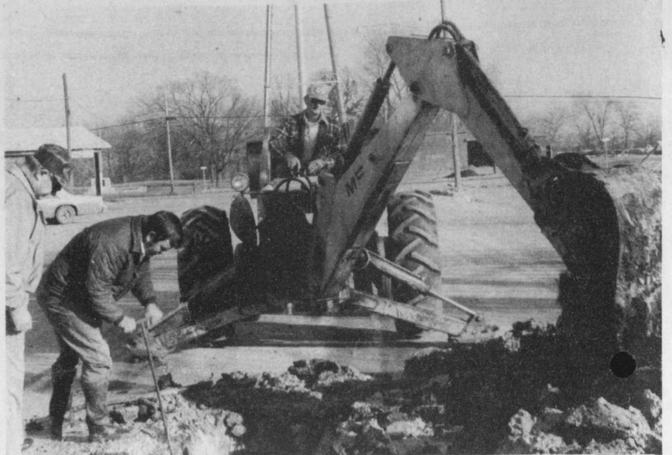
REPAIRS -city employees took advantage of a warmer day this week to begin repair to a leaking water line which was located directly in the center of main street in downtown Deport. The work required excavating a large hole in the middle of the street. (Staff Photo)
