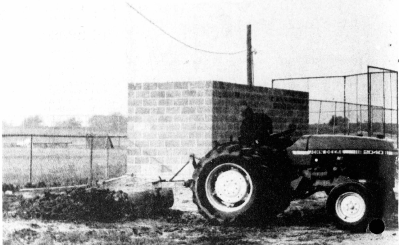
DUGOUTS-Work continues on the dugouts at the Prairiland baseball field at the high school. Concrete block dugouts and a water system at the pitcher's mound will add class to the Prairiland game! (Staff Photo)
