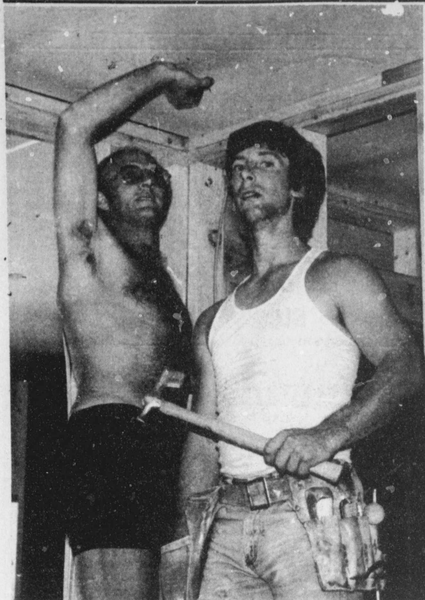
FIREMAN Doug Cato helps Johnny Dawson from Watson Dawson Drywall complete the sheetrock job on the Blossom Fire Station. They hope to have the job completed by the 22nd of July for the Fire Department's Jamboree. (Staff Photo)
