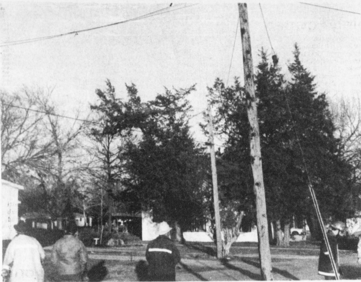
BALLS of fire shot down these power lines after something, or someone broke a line. The two high voltage lines touched as the
