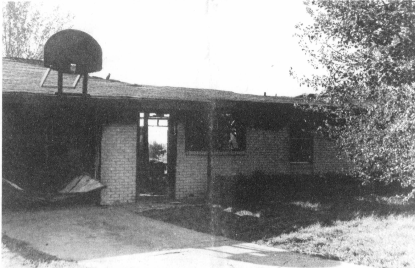
DESTROYED —The home of Sondra Annette was totally destroyed by fire of an unknown origin
