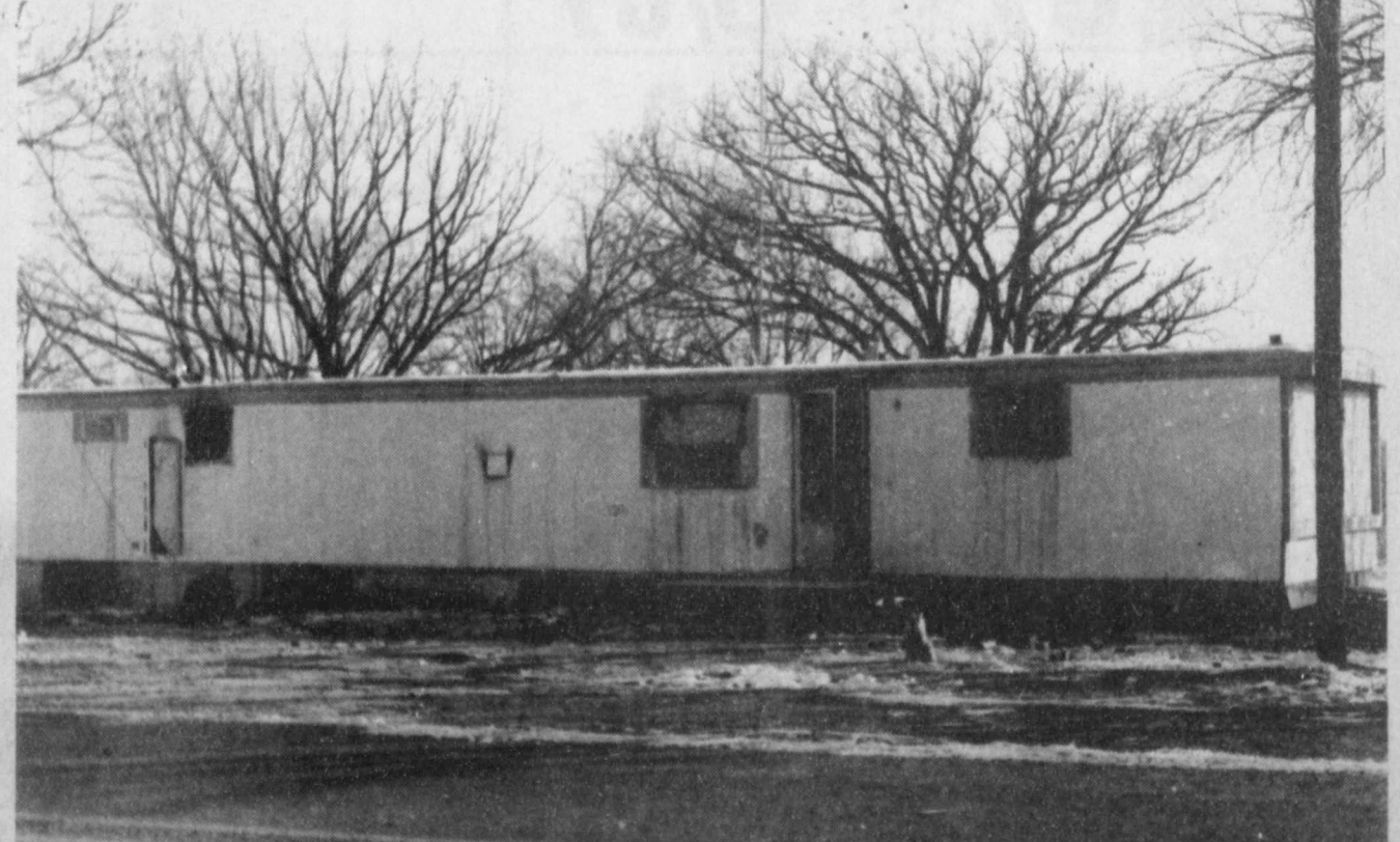
GUTTED—This mobile home, located in Pattonville, was destroyed on the interior by fire last Friday night. Members of the Deport Volunteer Firemen extinguished the blaze. The family occupying the home was named Smith, and had not been in the home for long. (Staff Photo)
