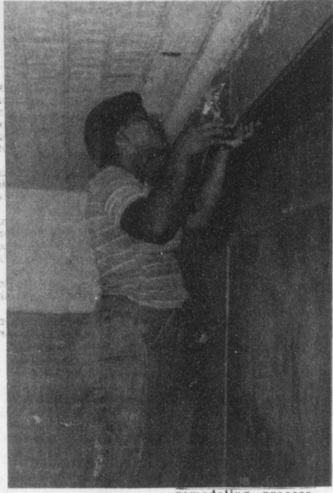
NIKKI WOOD-BERRY —is another eighth grade student working this summer at the Blossom School, helping with the remodeling process. Nikki is in one of the classrooms that renovation is being completed for the fall school term. (Staff Photo)
