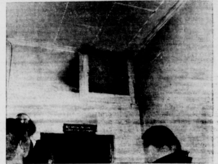
Smoldering fire, hidden from view of firemen, kept the volunteers busy long after the main blaze had been stilled. Here, firemen watch a suspect portion of the ceiling of the Boomtown Cafe, for further sparks. Cause of the blaze is unknown.
