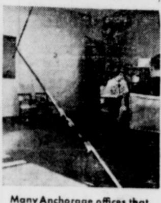
Many Anchorage offices that escaped destruction look like New York Life's, where steel braces are welded to pillars to help prevent further shifting of the building.
