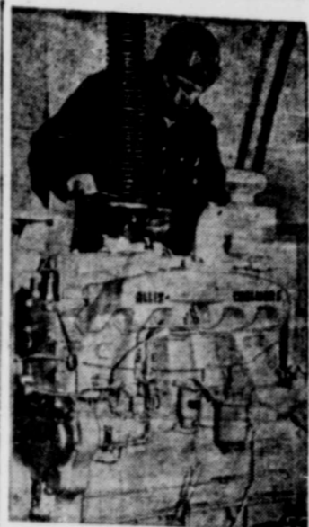
Jack Kasy, Minot, N. D., completes installation of Allis-Chalmers diesel engine-electric set inside a Minuteman missile launch control capsule.
