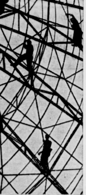
RESEMBLING CREATURES caught in a huge spider web, workers at Akron, O. construct radar tracking antenna for air force missile warning system.
