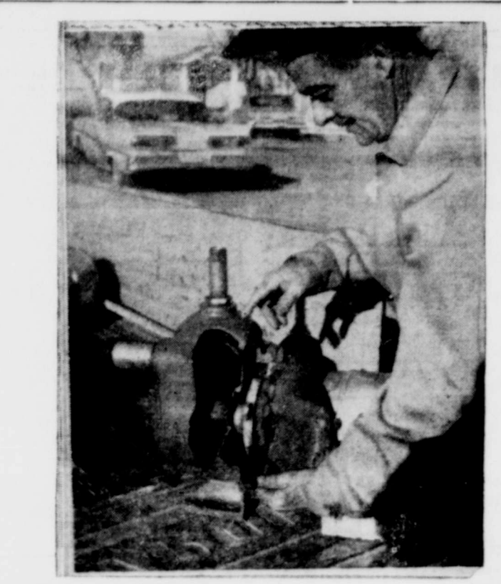
Shown above is one of the 15 water well pumps that froze during the recent cold spell when a momentary power failure was experienced. Haskell Draper, Water Superintendent, indicates the extent of damage to the waterwell pumps. Approximately $2,000 in repairs will be required to put the pumps back into operation.
