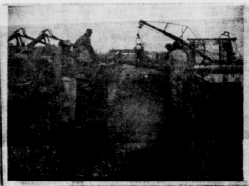
Water and Street Department crews join forces to get water line to the new Plastic Plant installed before weather turns bad.
