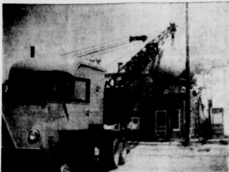
A crane lifting a milk storage, or cold wall tank to the top of the Preston Dairy building. This Cold Wall Tank will speed up operations by about 16,000 gallons a day, according to Buddy Prestor. Operating the crane is Larry Parks.
