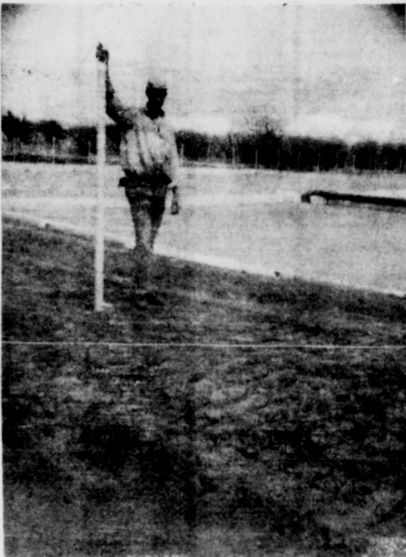
Installing fence around the new sewer disposal plant. In background are the Drying Beds of the plant.
