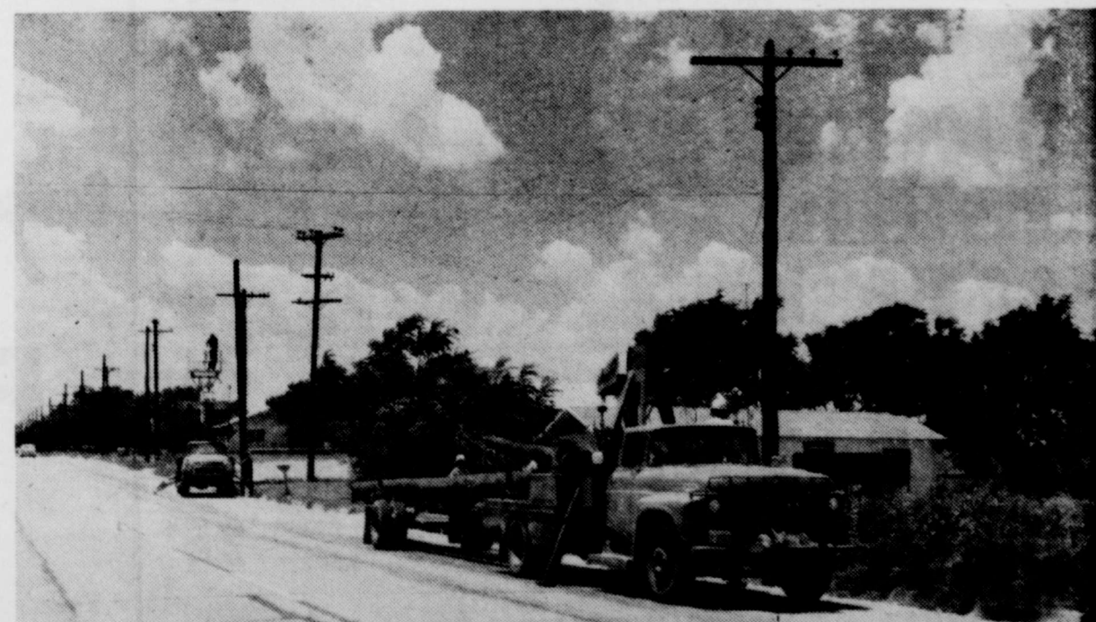
Poles are set for new 12,500-volt distribution line on West Third Street. Old 4,160-volt line is to be removed.
