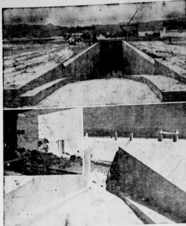
AUTO ENTRANCE ramp burrows inconspicuously into the desert as it leads down to a dual-purpose underground shelter and garage at the Operation Flumbob atomic tests in Nevada. Lower photo shows how the A-bomb blast crumbled part of the concrete retaining wall but failed to block the entrance. To the right of the crumbled wall is the entrance, closed by a 100-ton, four-foot-thick reinforced concrete blast door (inset), which was undamaged. (WTO Lookout Mountain Lab Photos)
