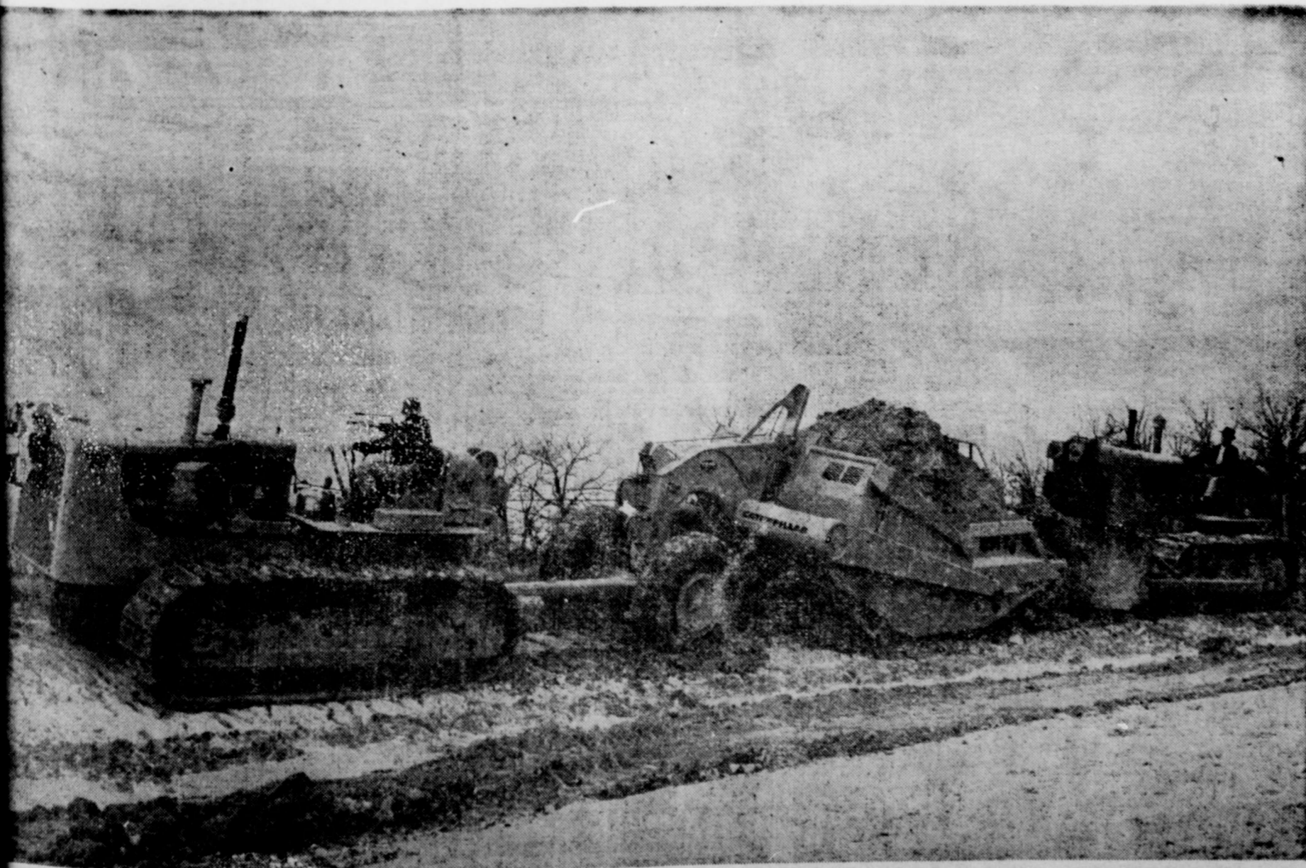
REAL PAYLOAD — Proper slope loading scraper operations are demonstrated during one of the Heavy Construction Equipment Operators Schools conducted at Texas A. and M. College by the Engineering Extension Service.
