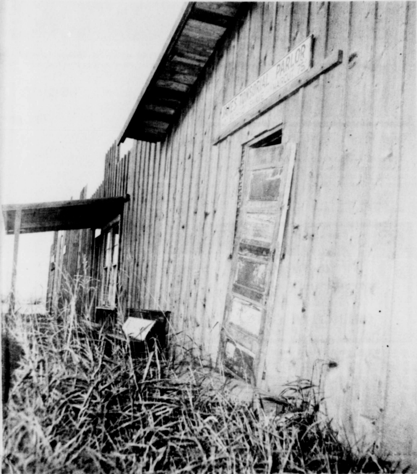
A photo of the "picturesque" Boomtown Oil Park in its present condition.
