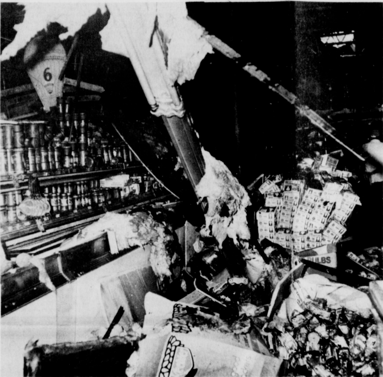
FIRE DAMAGE-- These related pictures depict a portion of the huge loss suffered by Piggly Wiggly as the Saturday night
