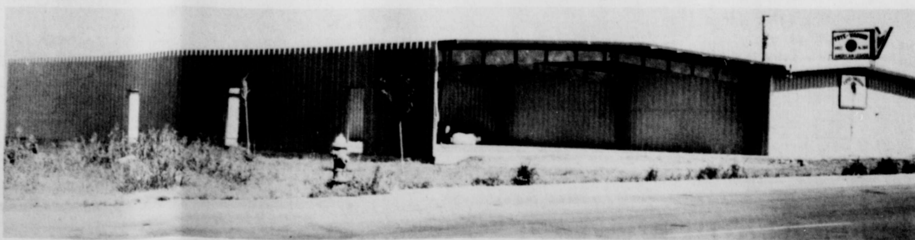
CONSTRUCTION UNDERWAY--American Legion Post 264 expansion in Burk Burnett has been underway recently. The old facility will have added to it a 60' x 96' structure which will be a main assembly room and will also house two offices and a stage. The old building (shown at right of expansion)
