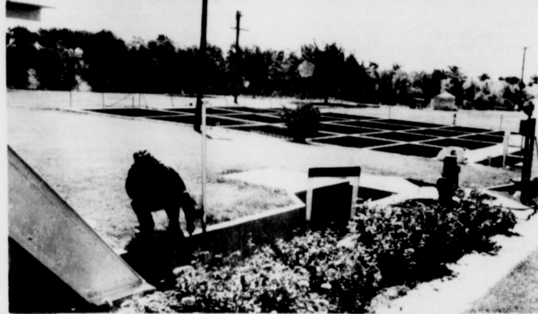
SHEPPARD AFB, TEXAS--WASTE TREATMENT--Airman Thomas Bewley checks the waste water as it first comes into the sanitation section's facilities south of the Sheppard Elementary School. The water will not go to the settling tanks in the background where the solid wastes will fall to the bottom. (USAF PHOTO BY AIRMAN LARRY ORR)
