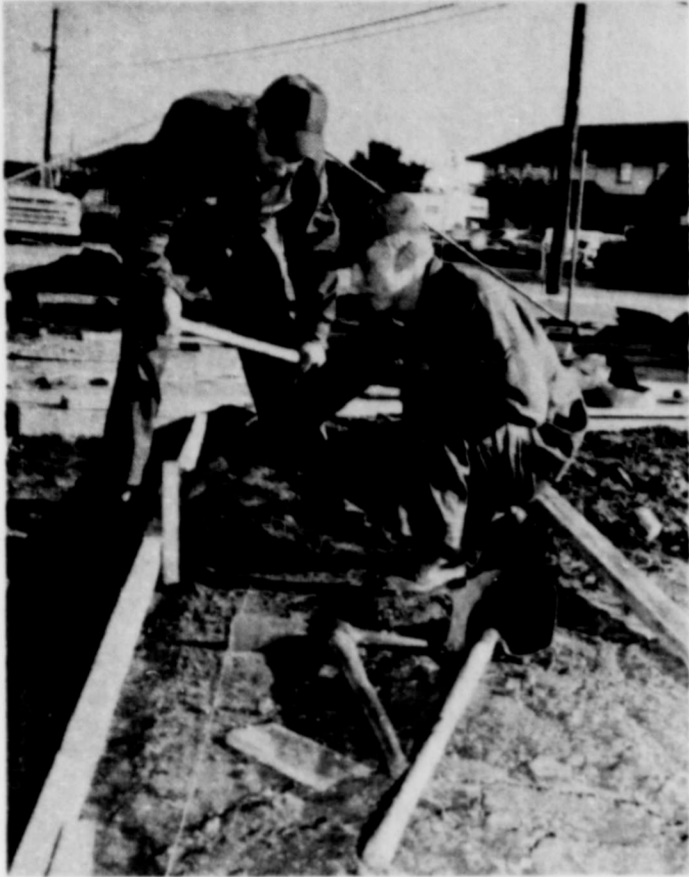
SHEPPARD AFB, TEXAS---SIDEWALKS--Airmen Richard J. Giers, left, and Robert O. Tucker, students in the Pavement Maintenance Course, Department of Civil Engineering Training, 3750th Technical School, build frames for pouring concrete sidewalks at the site of the new 12-hole miniature golf course at Sheppard AFB. Located opposite the Airmen's Club, the miniature links are a self-help project of the department, with funds provided by the Central Base Fund.
