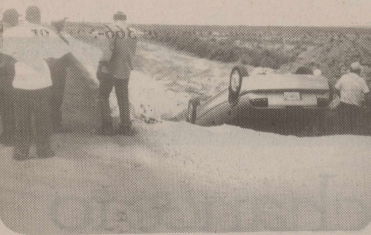
On Thursday, June 22nd-Monica Collier accidentally backed her car into a Culvert Preparation Hole. Fortunately no one was hurt. Collier, works for Highway Contractors out of Guymon, Oklahoma. This happened on the SE Corner of the Al Reznik Farm. (photo by Al Reznik)
