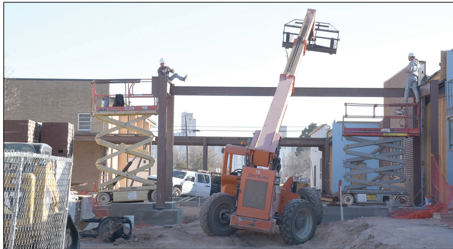
Construction of the new Primary School building is on schedule. Work has begun on the passageways that will connect the new building with the current Elementary School building across what used to be Cleveland Street.
