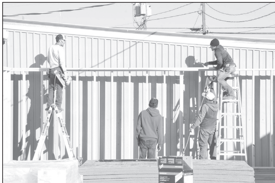
Before the winter blast hit, Trejo Roofing & Construction was busy putting up walls at the new Bookstore on the southwest end of the Friona Public Library. With good weather, the project should be finished near the end of April.
