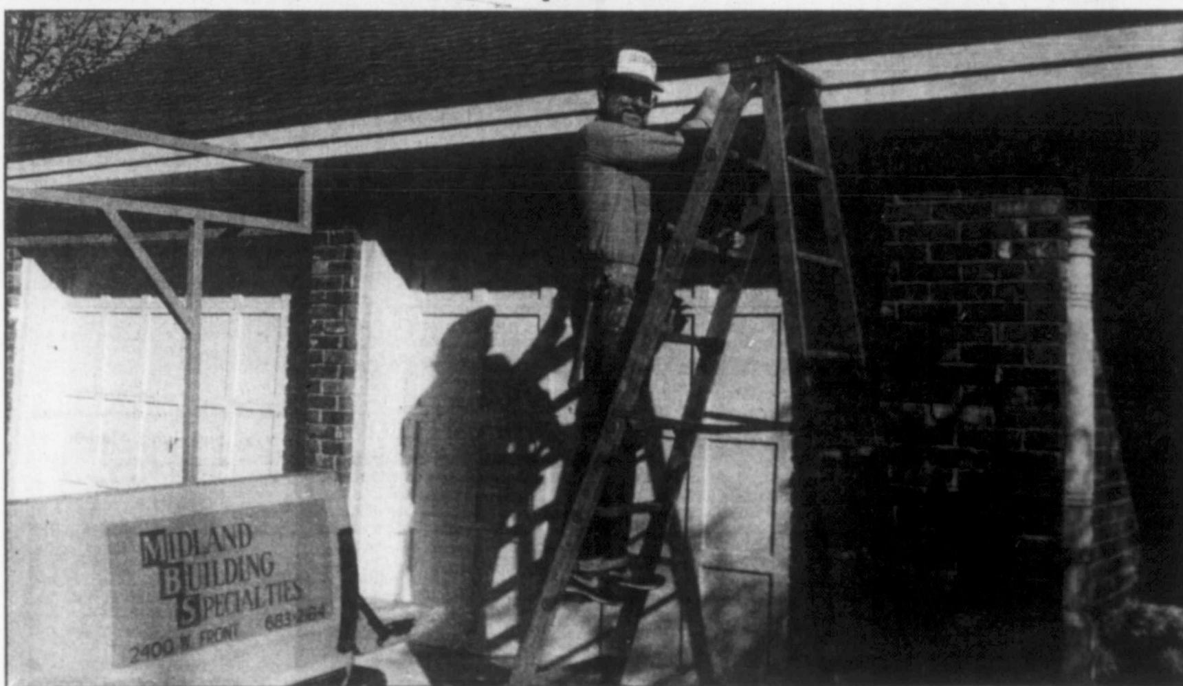
Jim Johnson of Midland Building Specialties finishes up the fascia on a recent soffit and fascia job. Call 683-2184 and find out what
