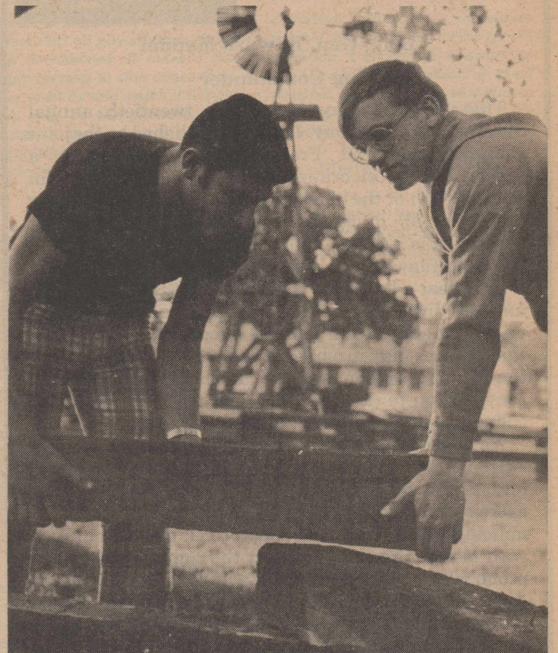
SPRING CLEAN UP—Robert Pisciotta (left) and James Guido joined 15 other people Saturday to put up railroad ties around Founders Park. The work is part of the continuing Spring Clean Up Campaign here. (U.S. Air Force Photo by SSgt. Ron Pack)
