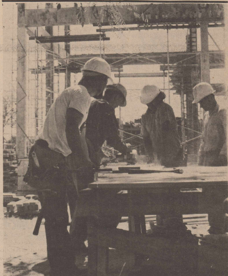
GOING UP — Work continues on the Reese Flight Simulator Building, which is now about 14 per cent completed. The simulator building, the first of its type in the Air Force, is scheduled for completion by July 1976. Equipment installation will begin at that time, with the facility scheduled to be fully operational by June 1977. (U.S. Air Force Photo by Sgt. Buddy Lerch)
