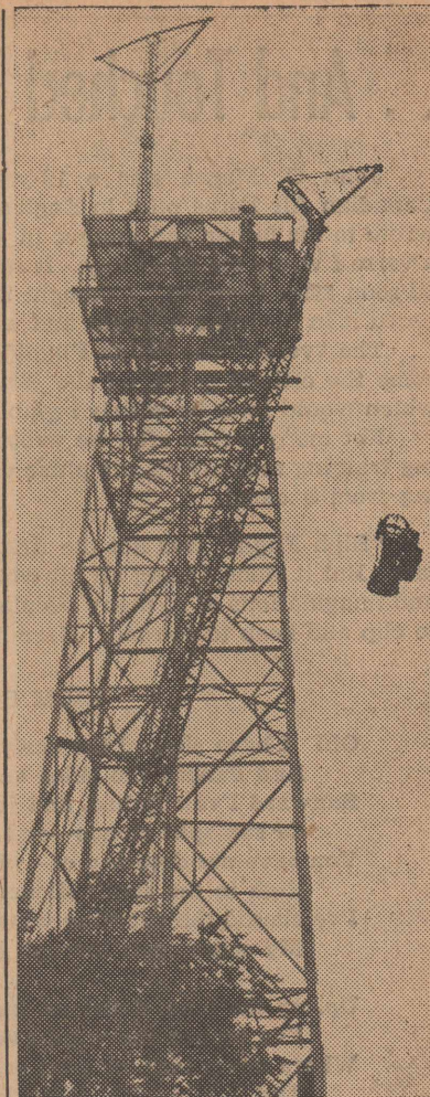
STORM WARNING TOWER — A radar unit is raised into position at the top of the recently constructed 100-foot steel storm warning tower, bringing the operation of the unit one step closer. In the next few weeks further equipment necessary for the operation of the warning system will be installed to complete the unit. The radar equipment will detect elements of a storm 60 to 100 miles away. (Photo by Bernard)
