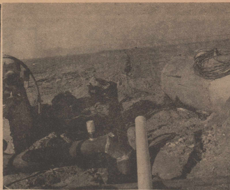
On the Johnny Jones farm, three light-producing wells are tied into one system. In this picture a four-inch plastic line is seen being hooked in at another well and then a six-inch line going to the overhead sprinkler system in the distance.
