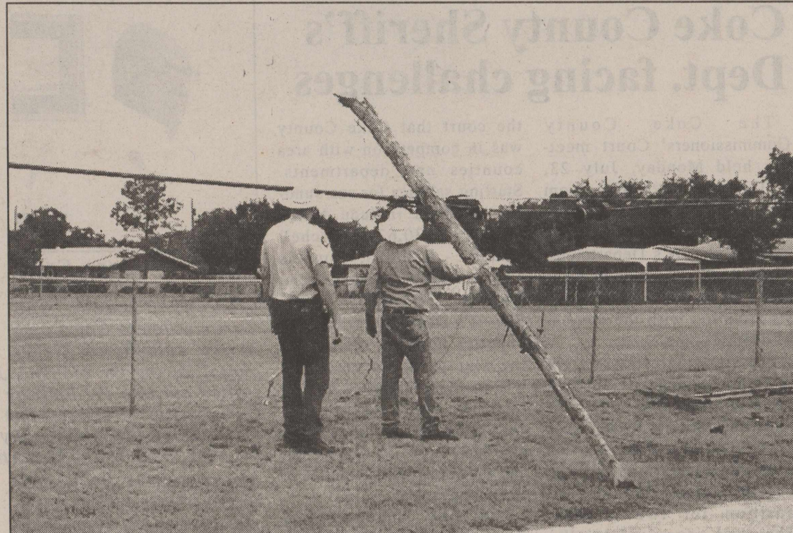
Pole Down! Coke County Sheriff's Deputy Adam Richter and AEP worker Wade Stautzenberger survey the damage of a down utility pole this past Tuesday morning. A delivery truck leaving Robert Lee ISD caught a sagging power line and accidentally pulled the pole down.
