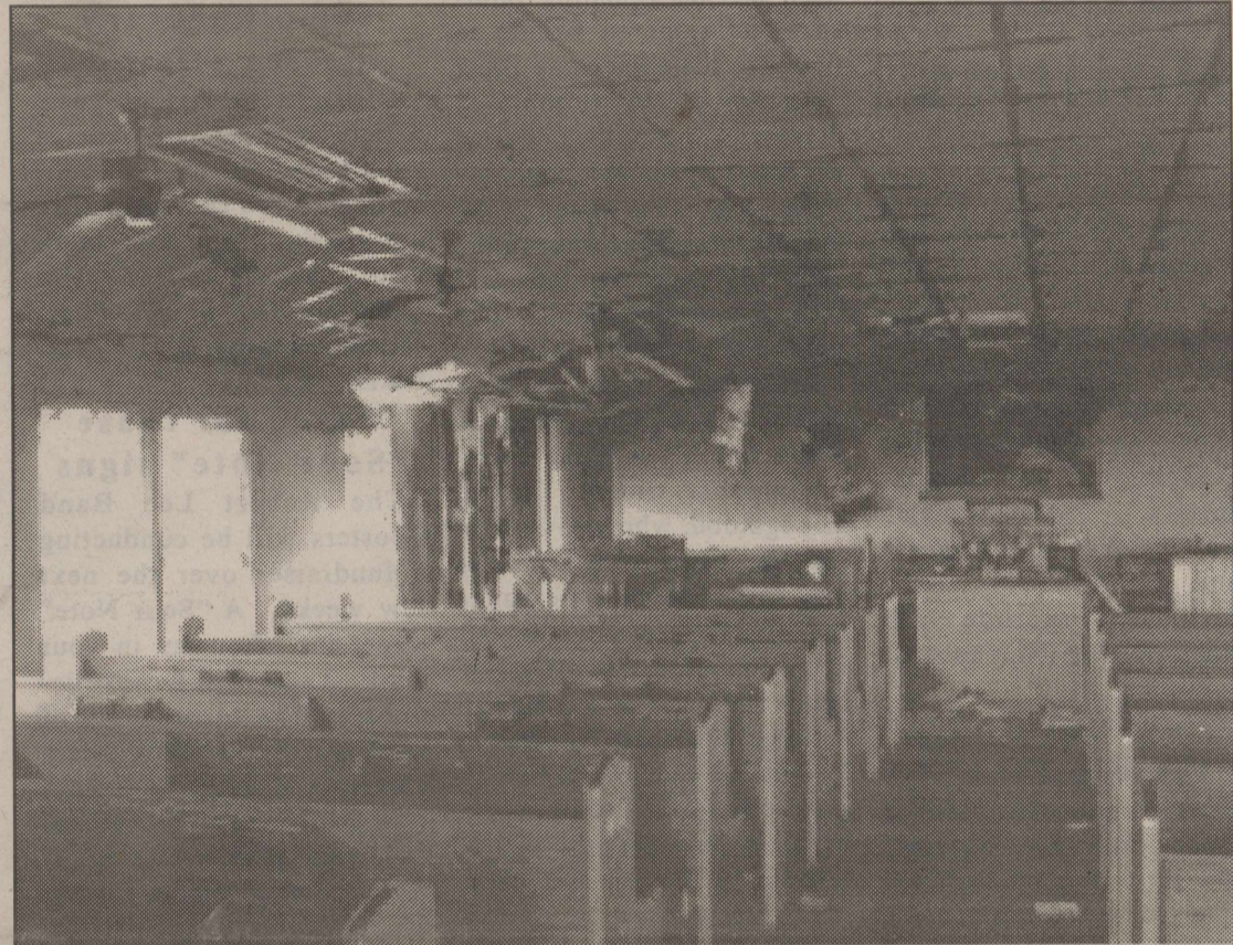
Fire at Pecan Baptist! At 4:15 am, Monday, October 9, Robert Lee Volunteer Fire Dept. responded to a call of a fire at Pecan Baptist Church. The fire began in the sanctuary by the piano next to the south entrance to the church. There was extensive damage to the interior, as shown by the above photo. Arson is suspected, as there was a window broken and signs of forced entry on the south side of the church annex. The fire is under investigation by the State Fire Marshall and the Coke County Sheriff's Department.
