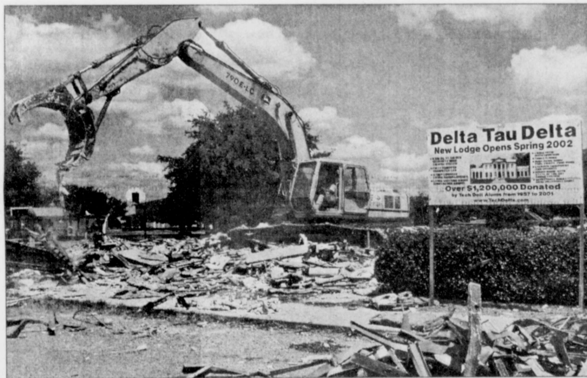
DAVID JOHNSON/Staff Photographer A WORKER WITH Matthews Backhoe demolishes the old Delta Tau Delta lodge on Greek Circle on Monday. The fraternity's new lodge, which has received more than $1.2 million in donations from fraternity alumni, is scheduled to open in Spring 2002.
