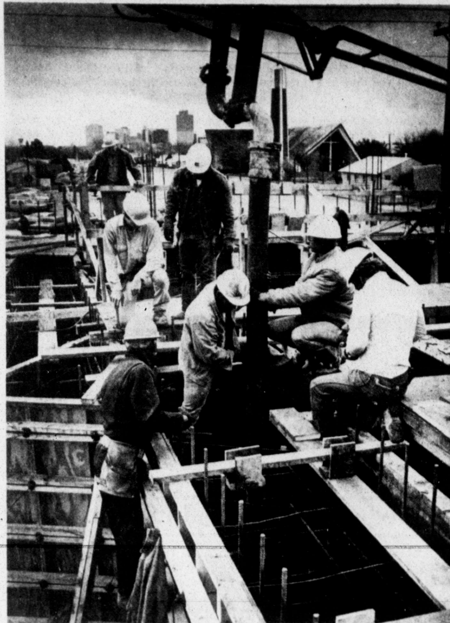
Workmen position equipment for Thursday's massive concrete pouring for the Allison Permian Basin Cancer Therapy Center. While more than 100 hospital officials and guests watched from an overlooking window in Midland Memorial Hospital, workmen poured 380 cubic yards of concrete into forms for six to seven foot thick walls around future radiation treatment rooms. The job took just over six hours. (Staff Photo by Brian Hendershot)
