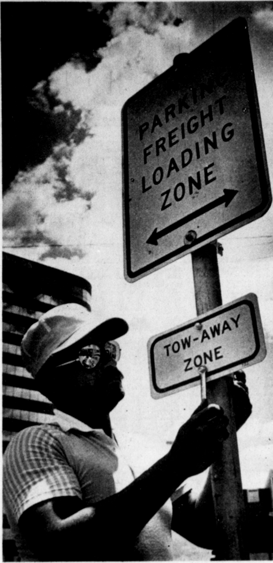
City employee Ruben Ramirez tightens the bolts on one of many tow-away zone, no parking signs installed Friday in downtown Midland. Police will soon begin enforcing the loading zone parking spots. (Staff Photo by Brian Hendershot)
