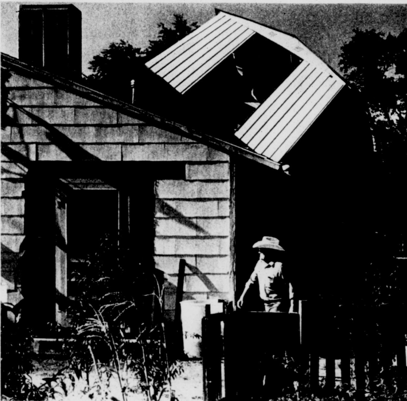
High winds Thursday added a temporary second story to a building at 701 S. Pecos St. occupied by Busy Bee Plumbing and Supply and the Midland Gem and Mineral Society. A metal storage shed
