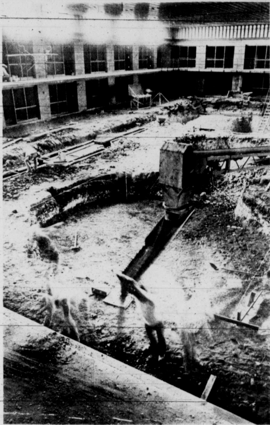
The ghostly figures in the foreground are construction workers pouring cement in the pool area of the new Holiday Inn, under construction on West U.S. Highway 80. The motel, scheduled for an Oct. 31 completion, will feature 205 rooms and banquet facilities for 1,600. (Staff Photo by Bruce Partain)
