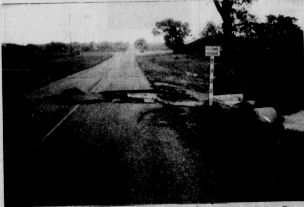
Damage to FM2731 due to water crossing over the highway near Union Center.
