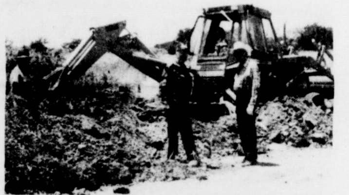
WATER FOR SCRANTON CENTER- Melvin Bailey, Nelson Geist and Jack Snoddy helping Johnny Ingram on the backhoe prepare for water lines to Scranton Community Center.
