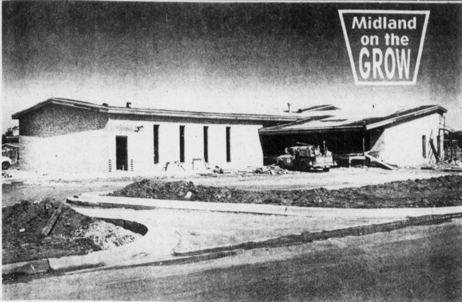
A new Salvation Army Chapel and Day Care Center is being constructed by Area Builders at 3500 Park Lane in Midland. Land for the building was donated by the Faskin Foundation and funds for the construction were raised by the people of Midland in a drive conducted especially for that purpose. The building will house eight classrooms, a multi-purpose hall and a 100-seat chapel. A fenced play area will be available near the building. (Staff Photo by Brian Hendershot)
