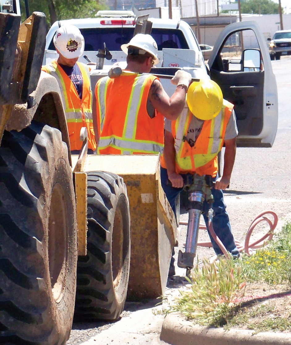
The signs say it all. Pictured above construction crews perform some of the preliminary work on West American Blvd., at 19th Street, Monday in preparation for the months of slower traffic and road construction with which local drivers will have to contend. Photographs by Larry Thornton
