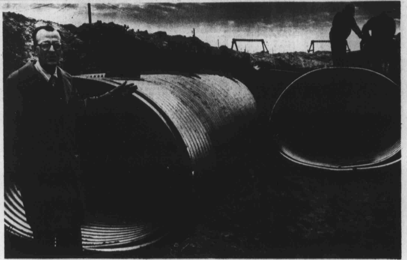
City Engineer George Medley points out the drainage pipelines being installed by the builders of Midland Park Mall. The mall's drainage will be
