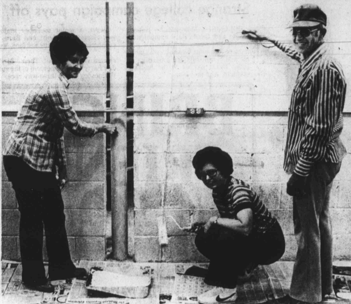
A fresh coat of paint is applied to the interior of the Mental Health and Mental Retardation Center on East U.S. Highway 80 Saturday by the Pioneer Club, a group of telephone employees who take on civic
