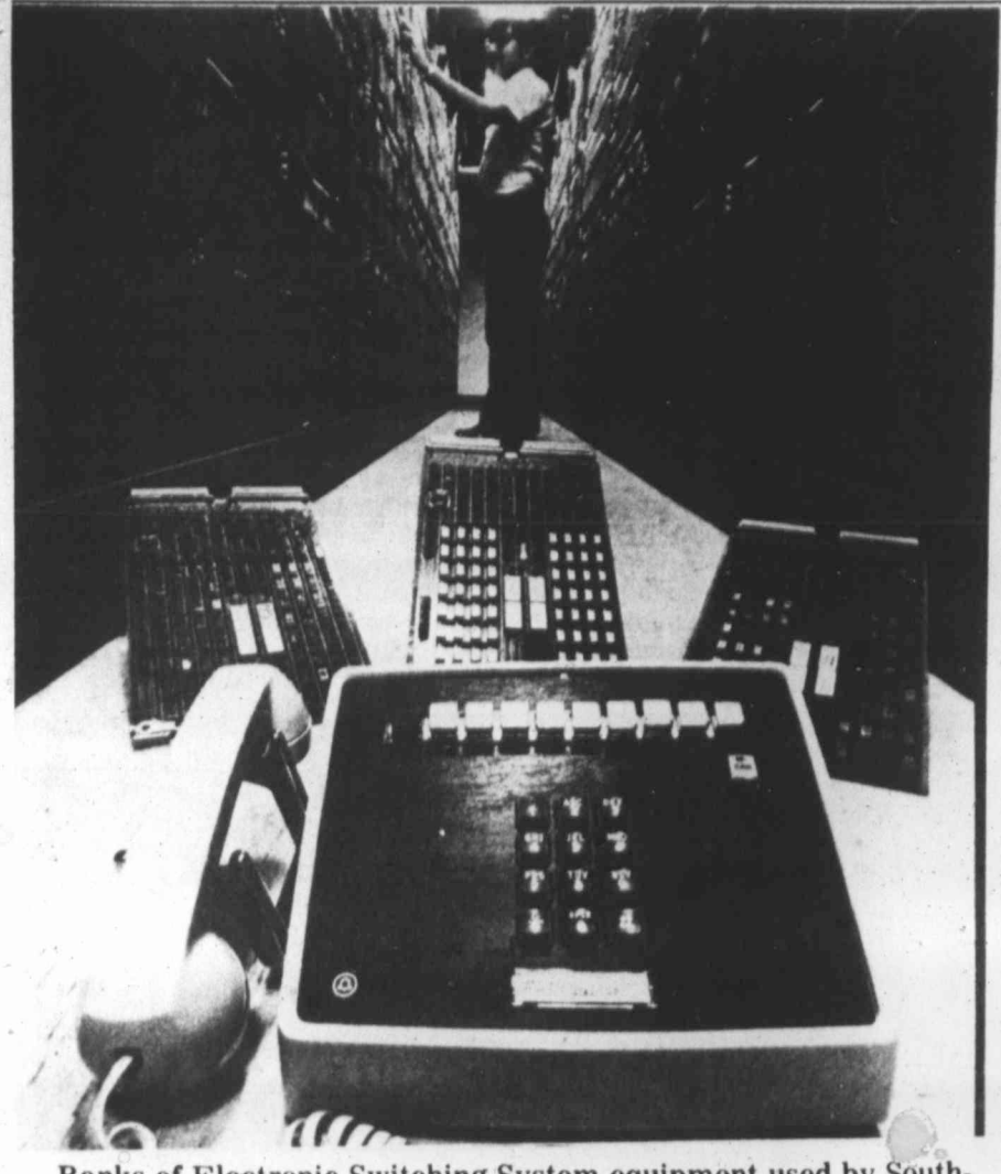
Banks of Electronic Switching System equipment used by Southwestern Bell Telephone Co. switch telephone calls in microseconds and provide custom-calling features such as "call waiting" and "call forwarding." The computerized equipment troubleshoots itself and alerts a technician when it needs help.
