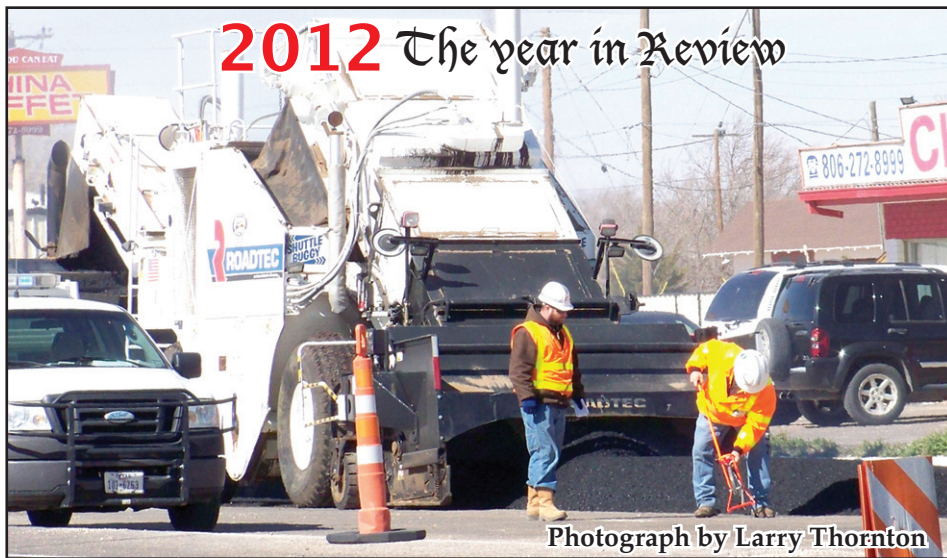
2012 The year in Review After months of preparation, asphalt was finally being laid on West American Blvd. in February, 2013.
