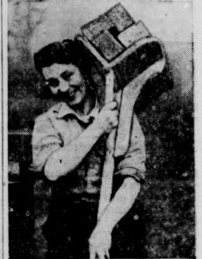
THE IRISH IN HER . . . Weary of waiting for official housing projects to get under way in Belfast, Ireland, Mrs. Joseph Close manfully shoulders a hod and totes bricks as she helps her husband build their own house.
