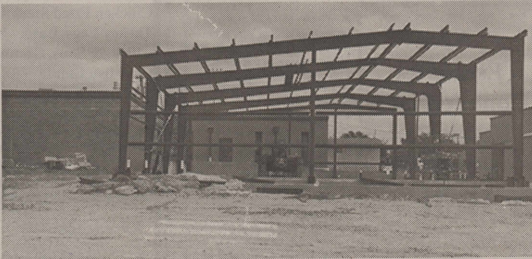
Progress on the new CPHS Band Hall. The new building is located between the elementary and high school buildings
