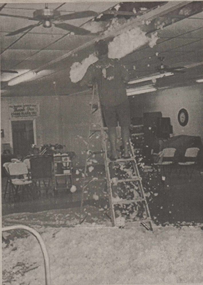
And the Insulation Falls Like Snow - Removing the Ceiling Tiles and Insulation was a messy job at the Senior Center. Photos from the remodeling on page 13.
