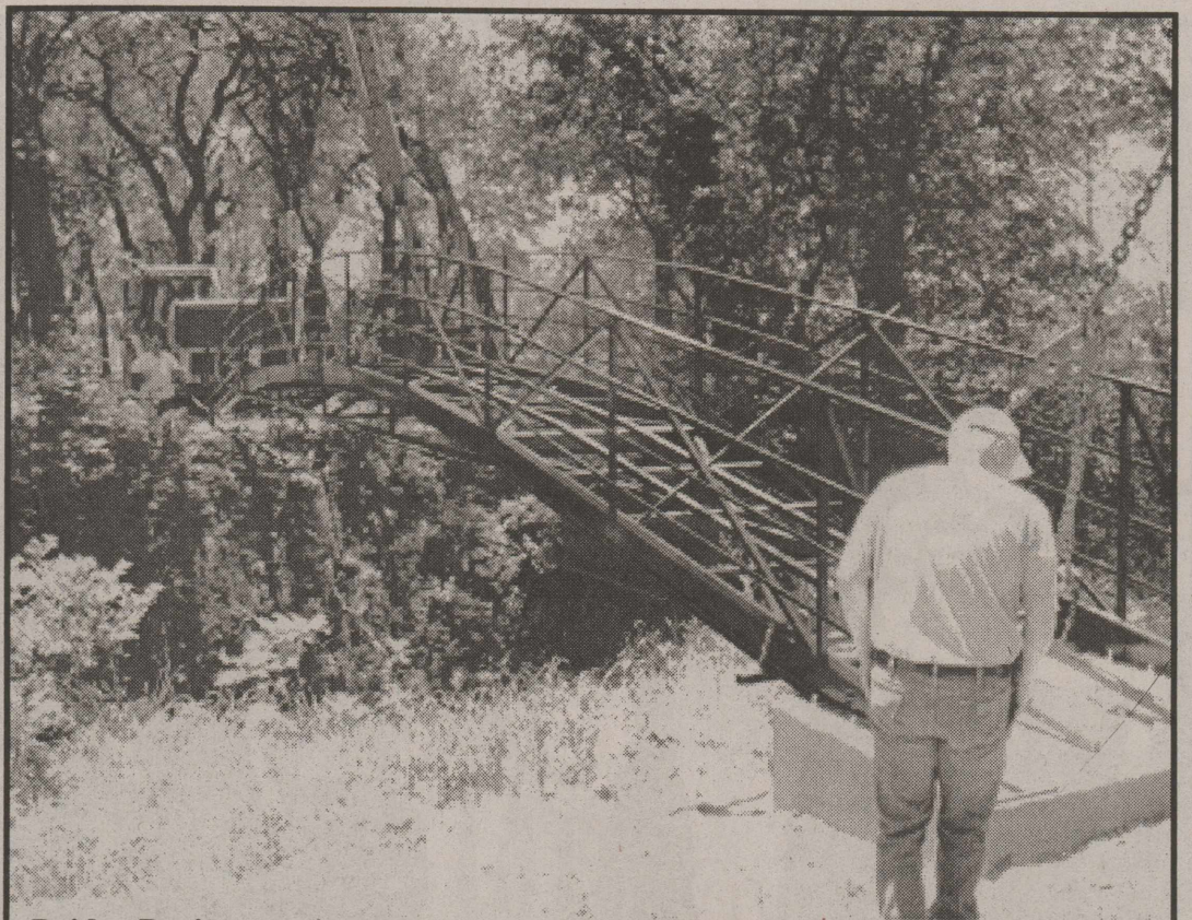
Bridge Project coming together quickly and nicely — Ken Horan, Mark Norris, Bo Allen, Brandon Blankenship and Doug Dugger set the Turkey Creek Bridge in place on Monday. Other volunteers helping were Scott Byrd, Robert Simons, Frankie Hyles, Stuart Sowell and Rick Potter. Volunteers will install the flooring for the bridge and finishing concrete will complete the bridge project in the coming weeks.
