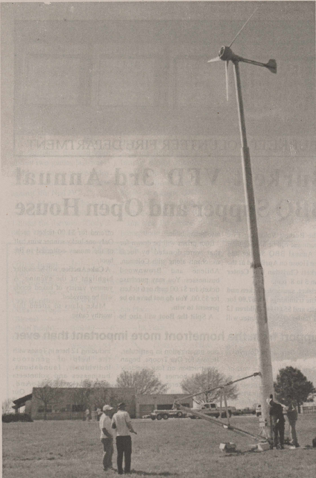
BLOWING IN THE WIND —Work crews from WeKnow Technologies and Evance look over the 60 foot residential wind turbine installed last Friday, March 25th at a residence on County Road 254, south of Clyde. The 5,000 KW wind turbine will power the 2,500 square foot home of Mike and Jenny Roetheli, pictured in the background. WeKnow Technologies, a master dealer and distributor for residential wind turbines, is located in Dallas. The wind turbine manufacturer Evance, is located in Loughborough, England.
